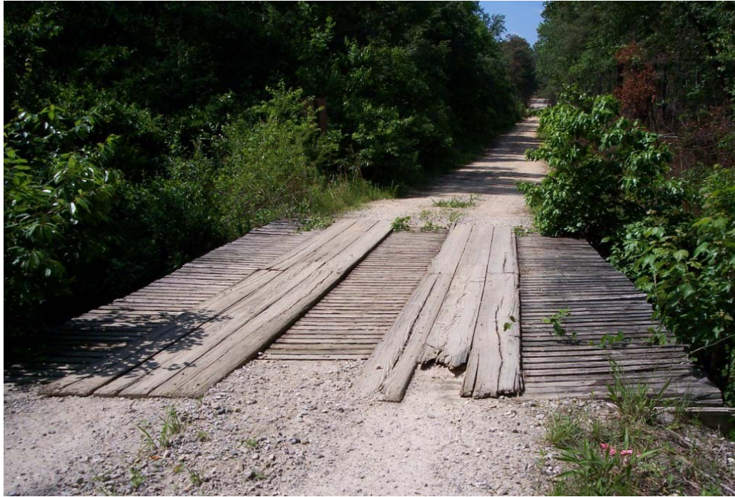
Figure 4. Original wood timber bridge at Fort Bragg to be replaced with thermoplastic composite bridge.
